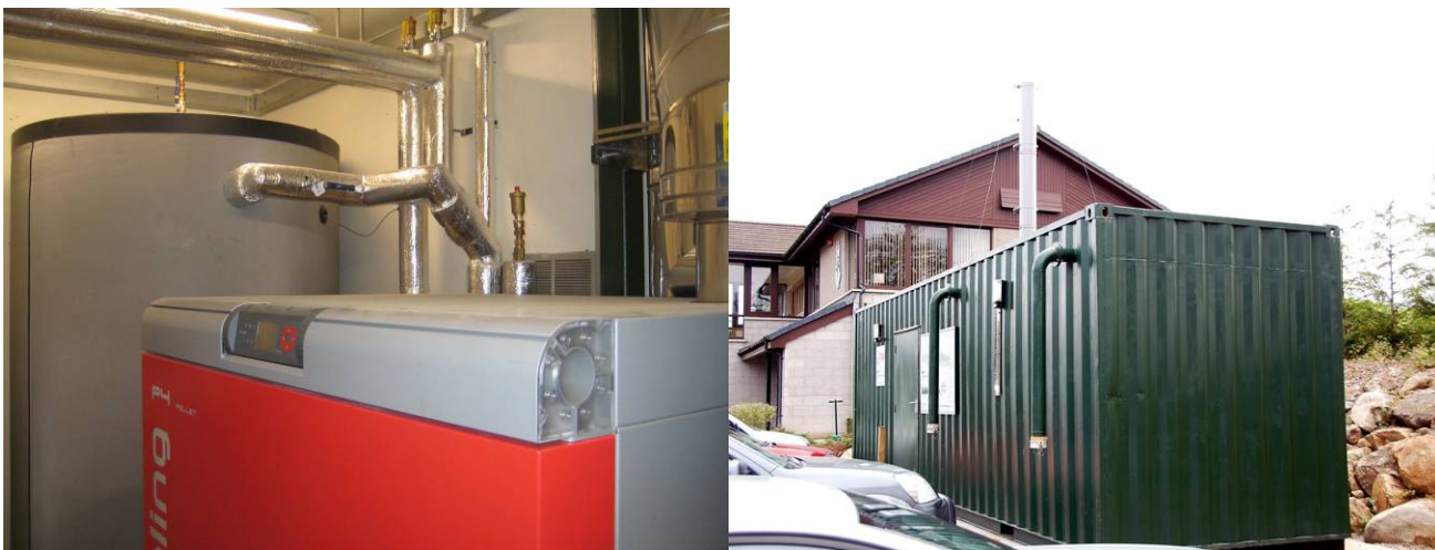
Biomass boiler and container
